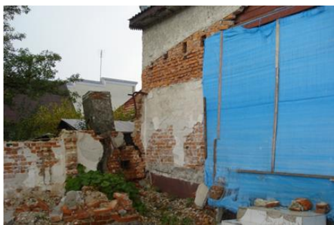
Figure 3.6.25: Partially collapsed house
