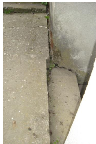
Figure 3.6.34: Gap between the basement staircase and the external wall
