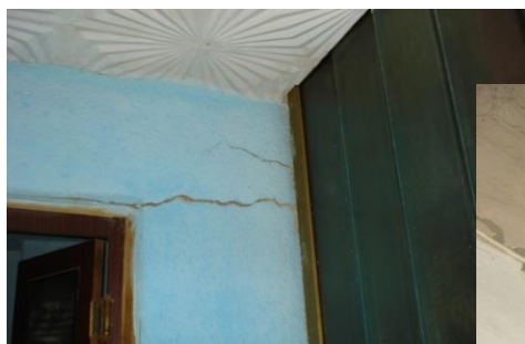
Figure 3.6.11: Through cracking on the masonry infill
