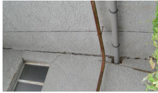
Figure 3.6.21: Masonry wall separated from the roof
