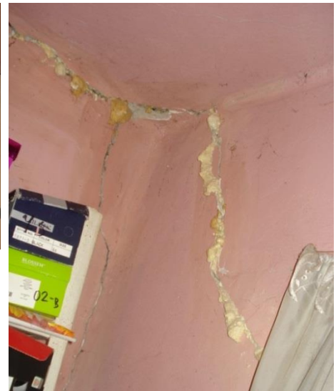
Figure 3.6.24: Extended through crackings
