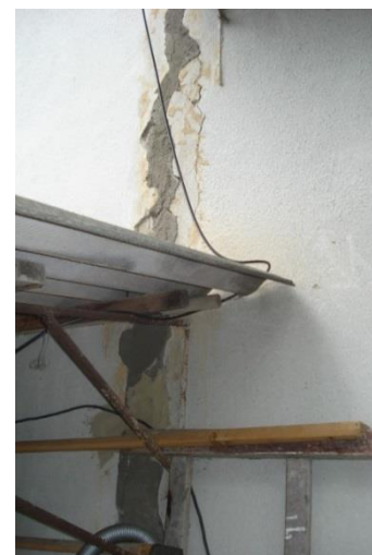
Figure 3.6.30: Vertical through cracking
