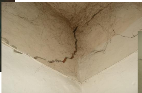
Figure 3.6.12: Extended cracking on the masonry
