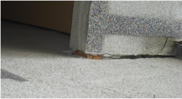
Figure 3.6.20: Masonry wall separated from the base
