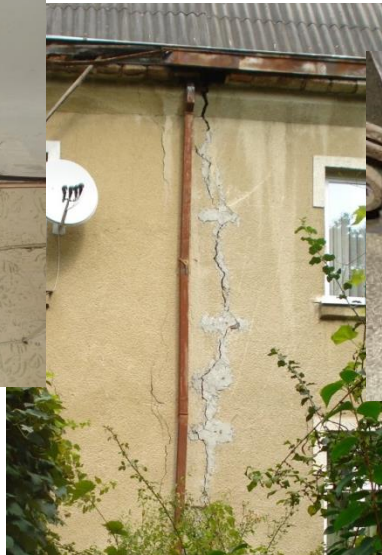
Figure 3.6.16: Vertical through cracking
