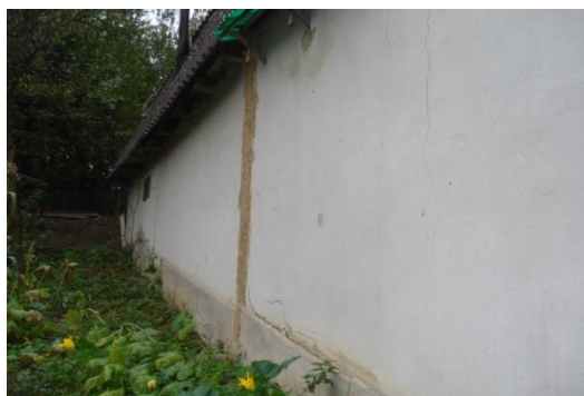
Figure 3.6.29: Vertical through cracking
