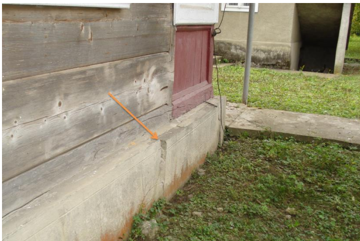
Figure 3.6.33: Cracking and obvious movement on the base of the wooden house
