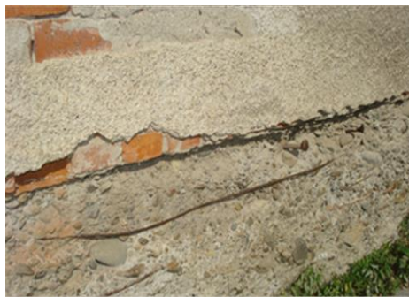
Figure 3.6.2: Poorly reinforced concrete platform
