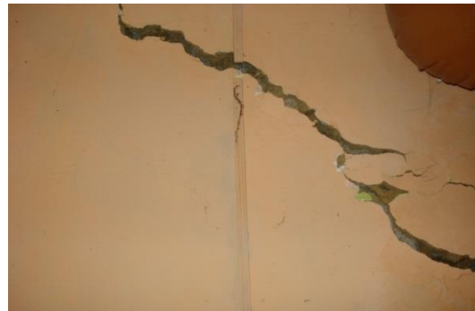
Figure 3.6.23: Extended through crackings
