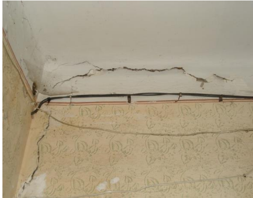
Figure 3.6.15: Internal masonry crackings
