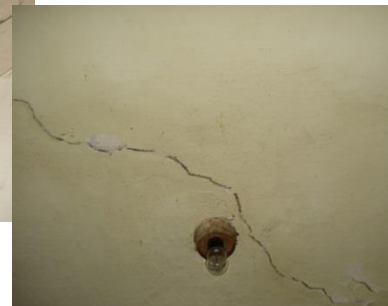
Figure 3.6.13: Extended cracking on the roof
