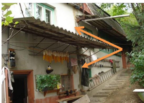
Figure 3.6.31: Vertical through cracking at the back side of the house
