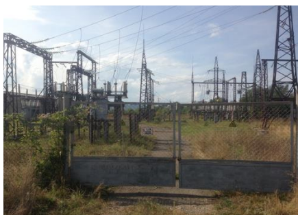
Figure 3.6.38: electric power substation
