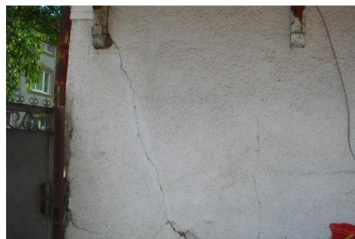
Figure 3.6.26: Through crackings at a house in the north side of Solena Street
