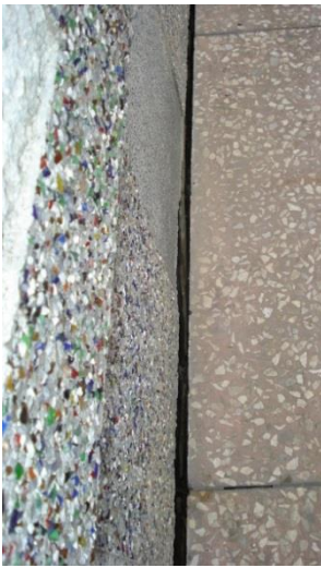
Figure 3.6.22: Gap between external wall and pavement
