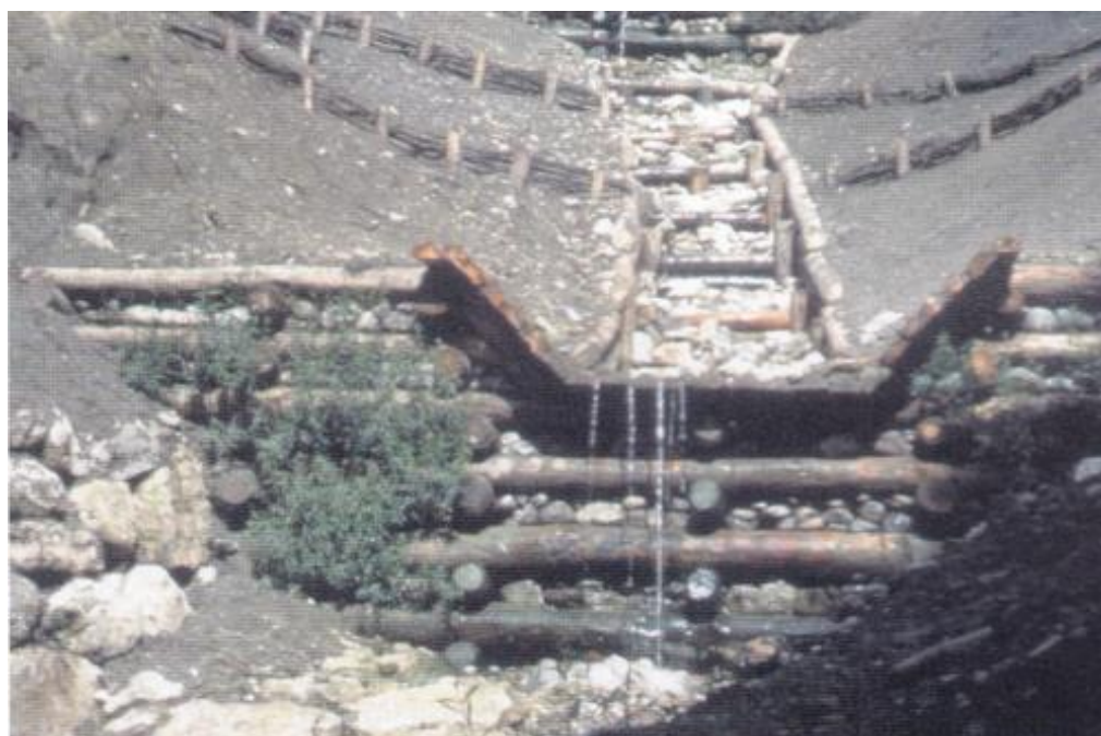
Figure 39 Erosion protection intervention using wood and stone (Malaguti 1993)
