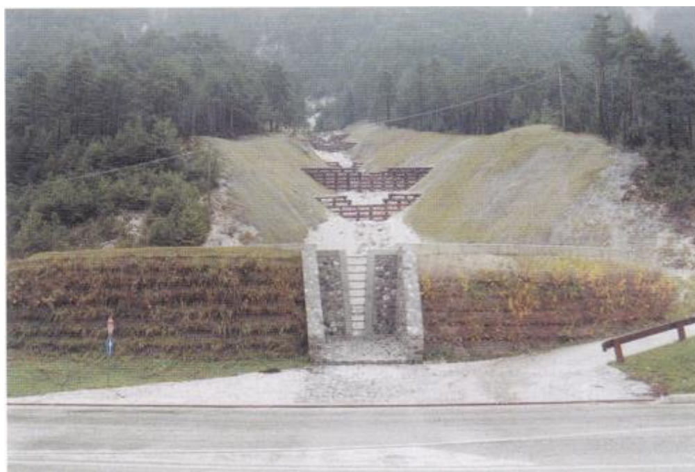
Figure 38 Wood and stone sediment trap dam and slope reduction dams (Malaguti 1993)
